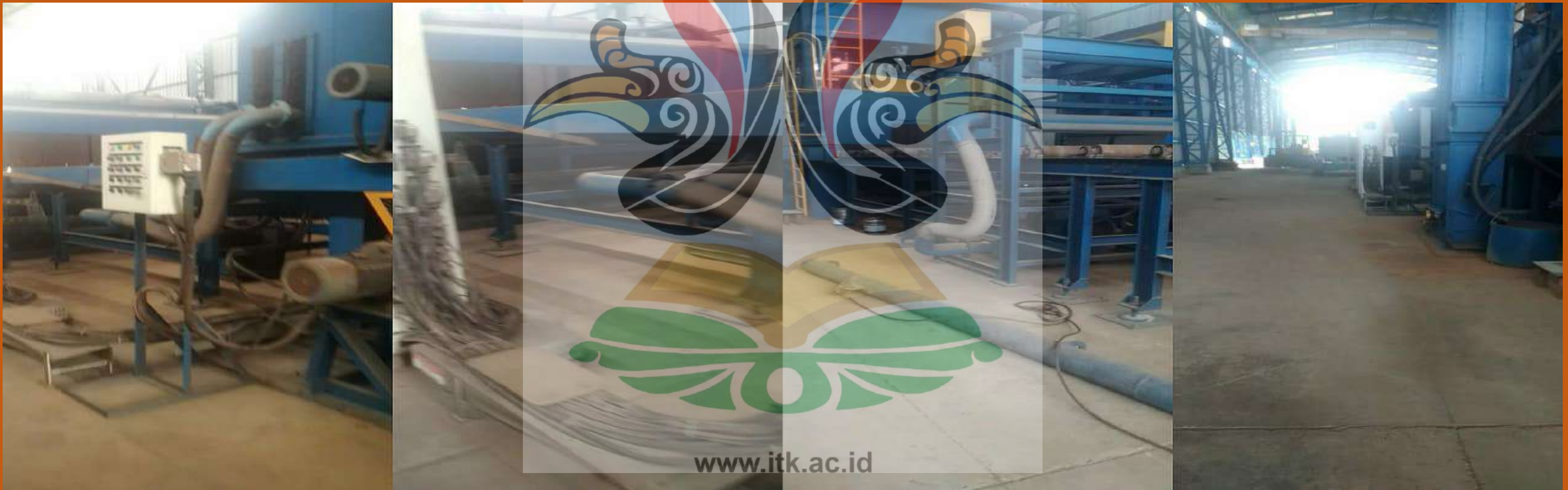
Gambar 4.2 mesin steel treatment plant
